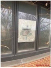
Left front window cracked/damaged and secured with
