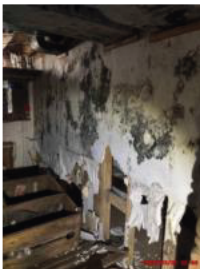
Discoloration on the basement drywall
