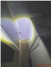
Discoloration im rear bathroom
