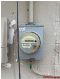
Photos - Electric Meter (limit 4) *
