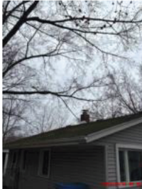
Roof has moss on both sides.
