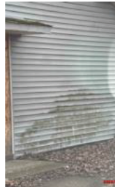
Moss build up on t front of the property, all sides
