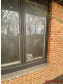
Left front window cracked/damaged.
