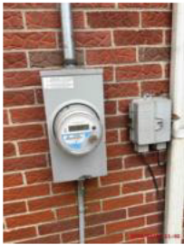
Photos - Electric Meter (limit 4) *
