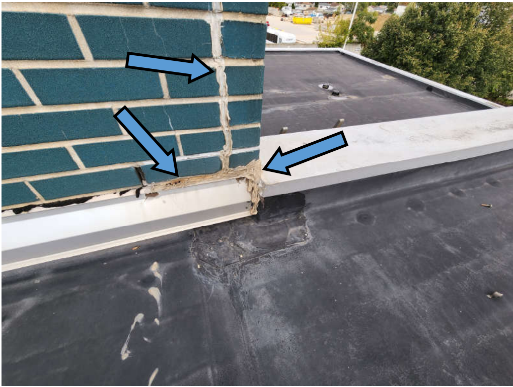
Above the copy room and office leak (which are the same) the wall is in poor condition with multiple repair attempts made with caulk.
