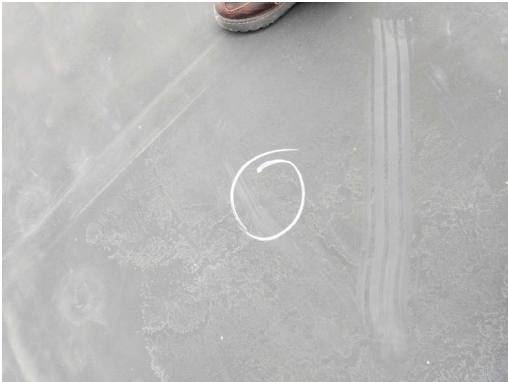
Puncture in the roof over the computers.
