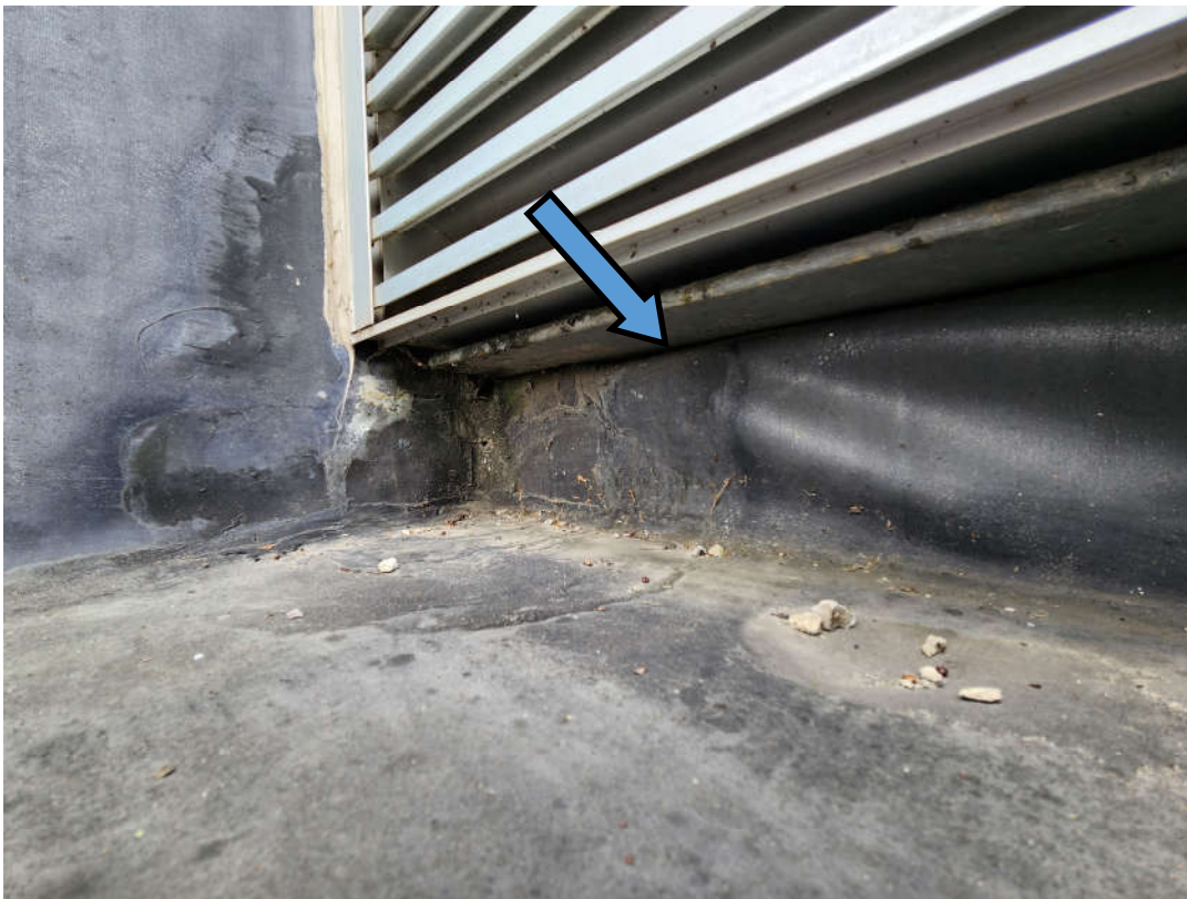
Flashings are extended up and under the low curb along the wall vents. This will need redesigning when roofing is replaced.
