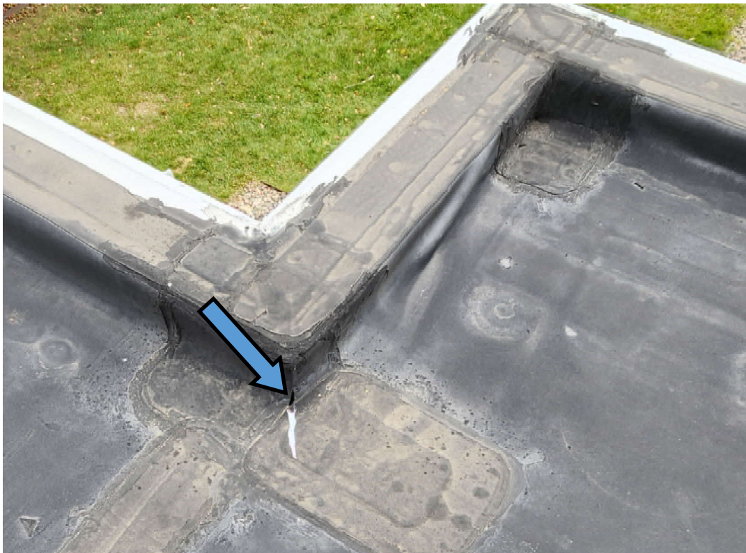
Deteriorated and open corner flashing on the low north roof area.
