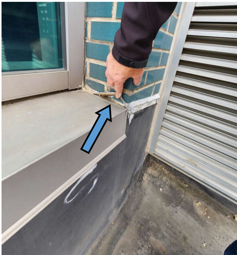
Failing sealant above the office leak.
