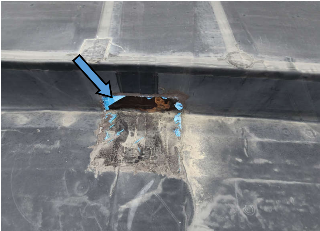
Miscellaneous repairs have been improperly attempted with asphaltic materials on this EPDM roof.
