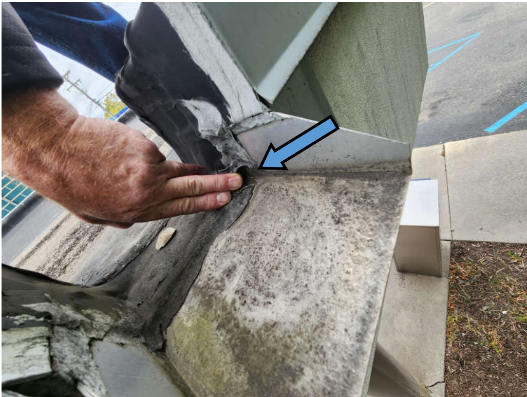
Failing scupper flashing on the low entrance roof.
