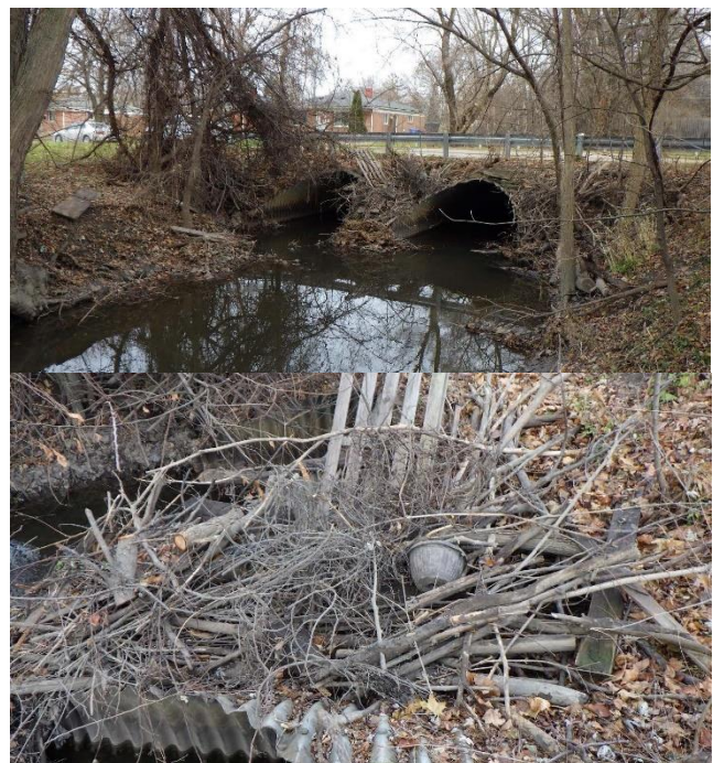
Figure 3: Debris catch at Polk Street
