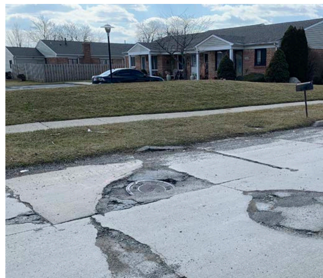
Previous State of Disrepair
