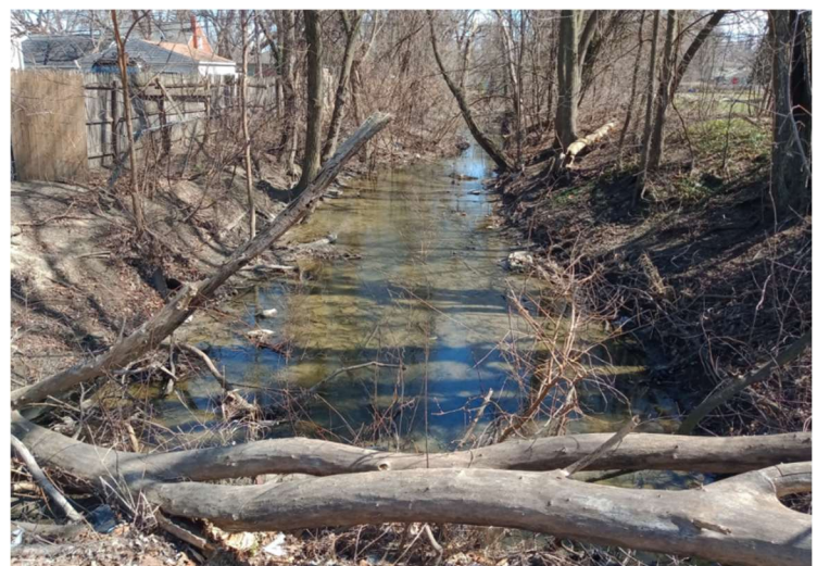
2-Debris buildup at culvert
