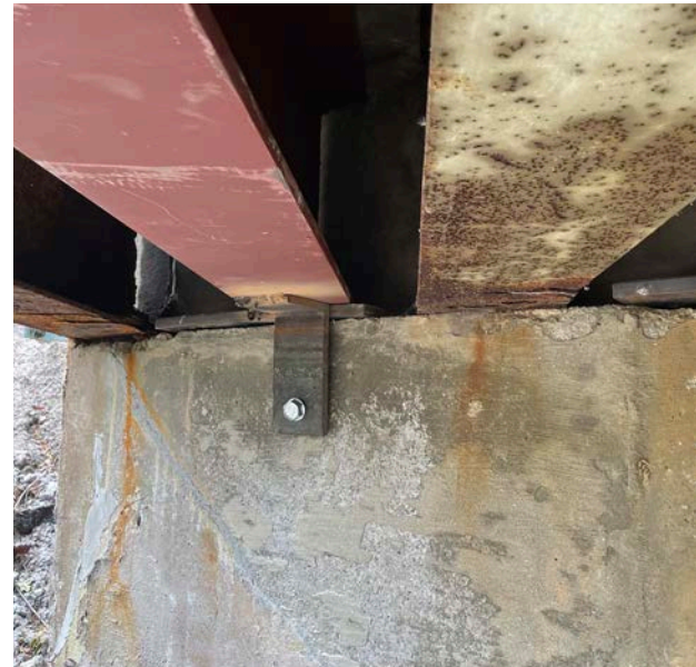
Previous Wear Under Bridge
