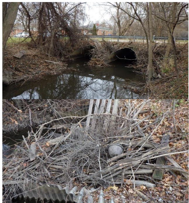
Figure 3: Debris catch at Polk Street
